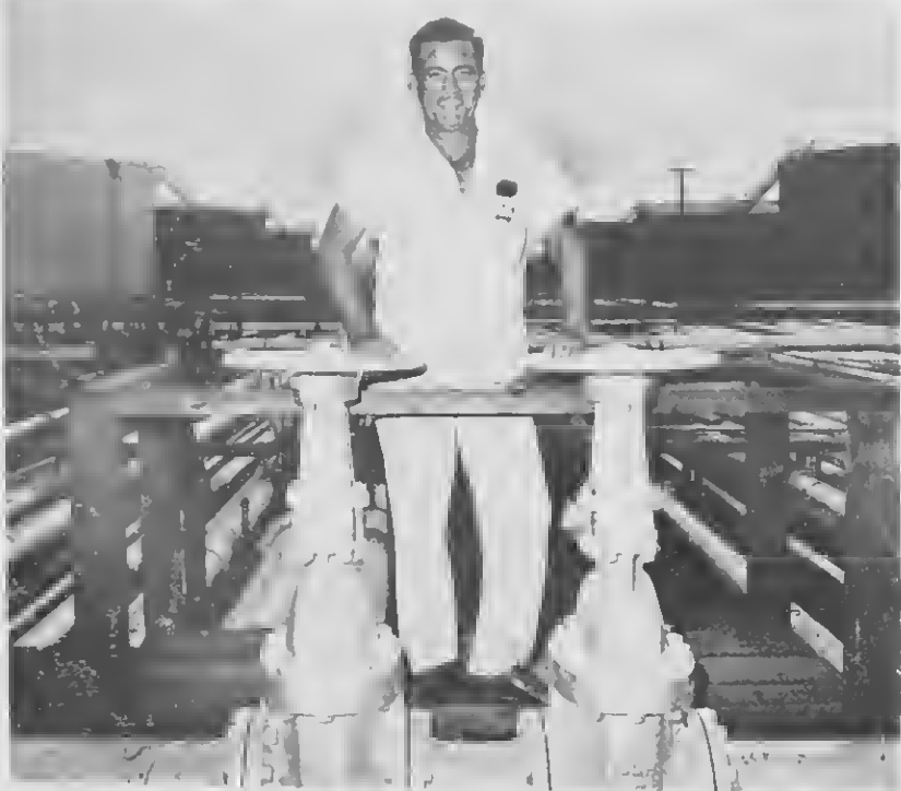
A Fls. 1000 winner poses by the main installation of his suggestion. Assistant operator in the Process Department, F. S. Kelly recently received a neat Fls. 1000 CYI check for his accepted suggestion that concerned pipe lines, time saved and availability of pumps.
